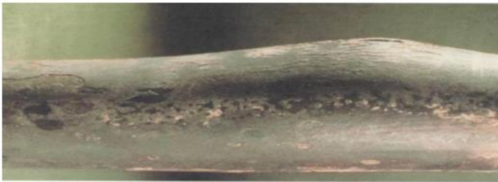
Fig.2-Tube failed due to high temperature
