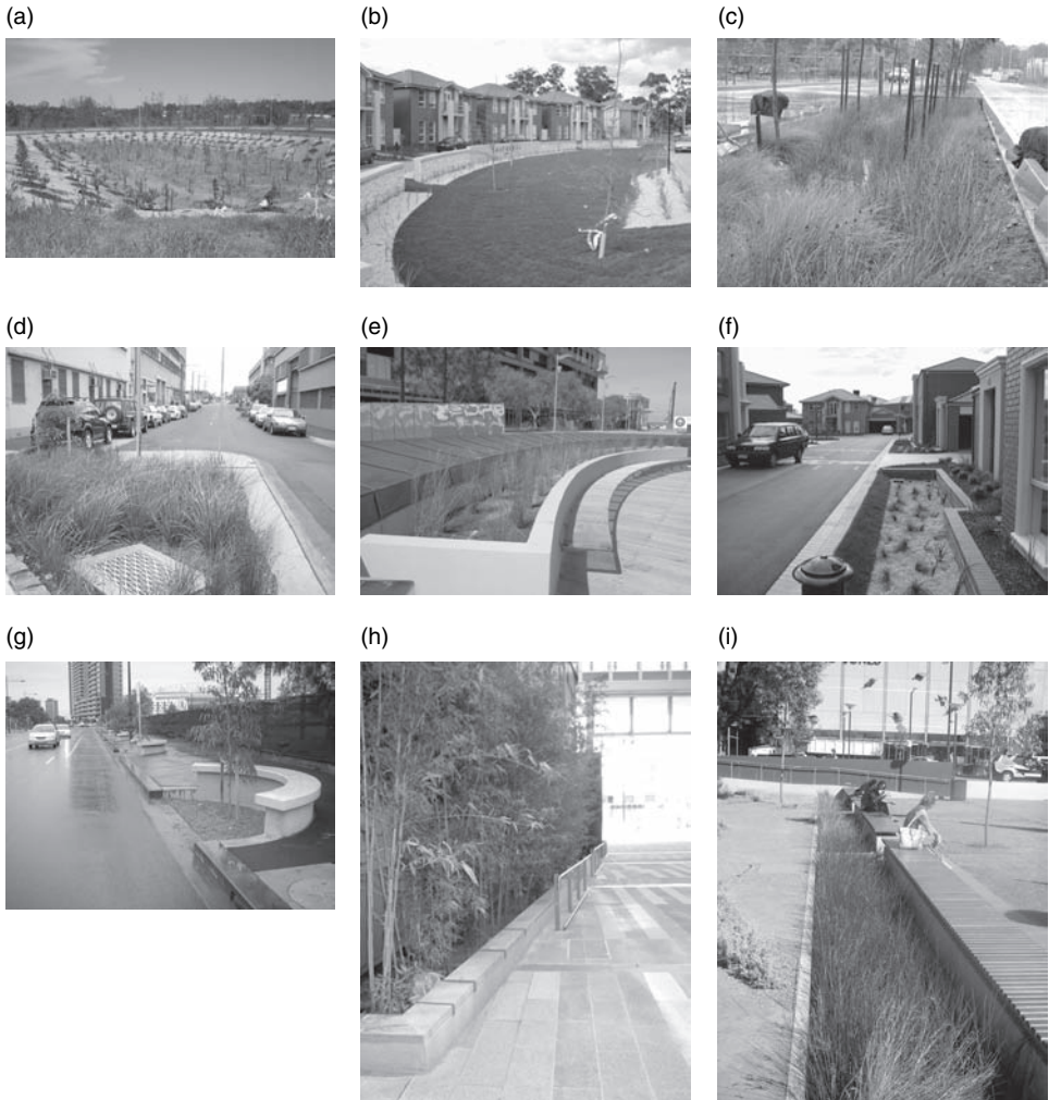
Figure 23.5. Stormwater bioretention systems recently constructed around Australia. (a) Hoyland Street bioretention basin, Bracken Ridge, Qld (engineer: Brisbane City Council); (b) Baltusrol Estate, Moorabbin, Vic; (c) Victoria Park, Zetland, NSW; (d) Cremorne Street, Richmond, Vic; (e) Victoria Harbour, Melbourne Docklands, Vic (Lend Lease); (f) Baltusrol Estate, Moorabbin, Vic; (g) Batman Avenue tree planters, Melbourne Dockland, Vic (VicUrban); (h) NAB Building, Melbourne Docklands, Vic (Lend Lease); (i) Adelaide Museum Forecourt.
