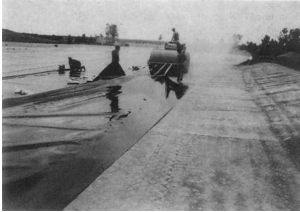
FIGURE 14.3 Geosynthetic fabric liner installation conforms to composite liner federal requirements for MSWLFs at the expansion site of Caldwell Sanitary Landfill. (Source: Caldwell Sanitary Landfill. With permission.)
