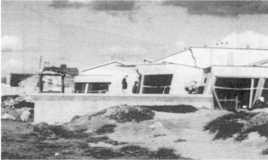
FIGURE 25.7 Liquefaction-induced damage of the Marina Research Facility at Moss Landing, California, caused by the 1989 Loma Prieta earthquake (after Seed, R. B., Dickenson, S. E., Riemer, M. F., Bray, J. D., Sitar, N., Mitchell, J. K., Idriss, I. M., Kayen, R. E., Kropp, A., Harder, L. F., and Power, M. S. 1990. Preliminary Report on the Principal Geotechnical Aspects of the October 17, 1989 Loma Prieta Earthquake. Earthquake Engineering Research Center, Report No. UCB/EERC-90/05, University of California).
