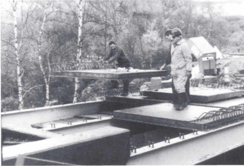
Fig. 8.2. Installation of open sandwich deck slabs on bridge south of Loch Tummel, Tayside.
