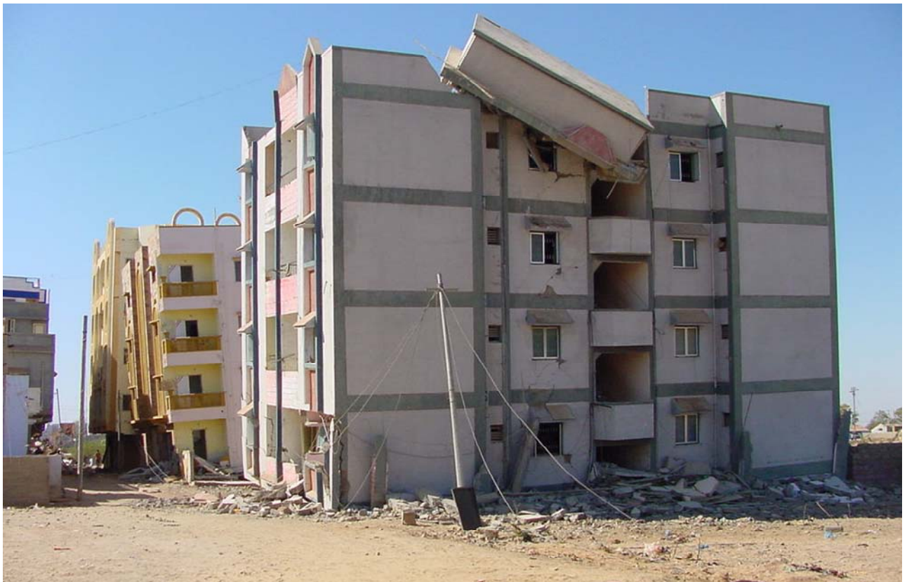
Figure 1.8: Failure of small capacity water tanks atop RC buildings during 2001 Bhuj (India) earthquake: they need to be formally anchored to rooftops, else they can dislodge from the roof
