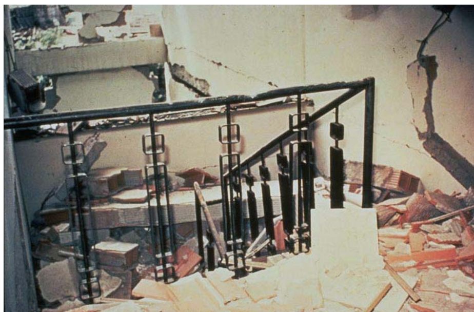
Figure 1.11: Undesirable earthquake performance of elements assumed to be non-structural elements during 1972 Nicaragua Earthquake: Damage to unreinforced masonry infill and floor tiles around stairwell (Photo: The EERI Annotated Slide Collection, 1997)
