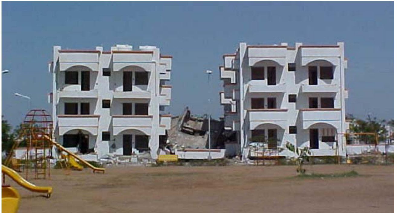
Figure 1.6: Collapse of one set of RC frame buildings during 2001 Bhuj (India) earthquake: there is relatively minimal damage in the stiff upper portion, while the lower storey is completely crushed. The almost identical building in the background is completely collapsed.
