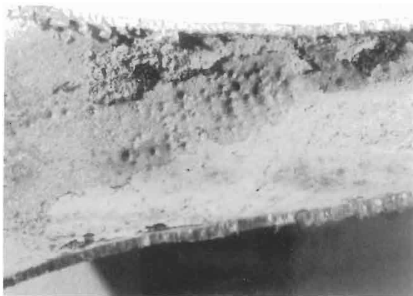
Fig. 3. The internal surface of a tube showing extensive pitting ( \times 3 ).
