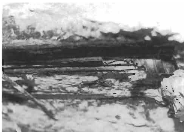
Fig. 3. Corrosion damage of cables.
