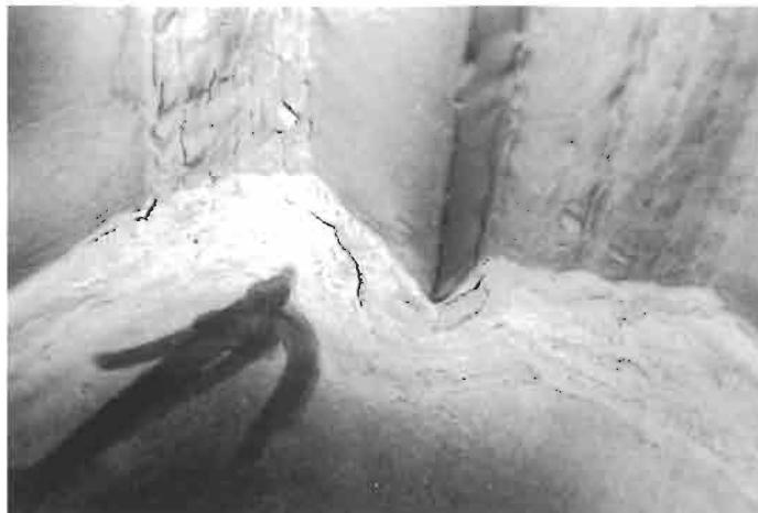
Fig. 4. Typical cracks found at external support welds.
